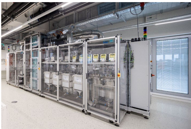
Powder-Up! Pilot plant for the production of active materials for sodium-ion batteries. © ZSW Ulm
